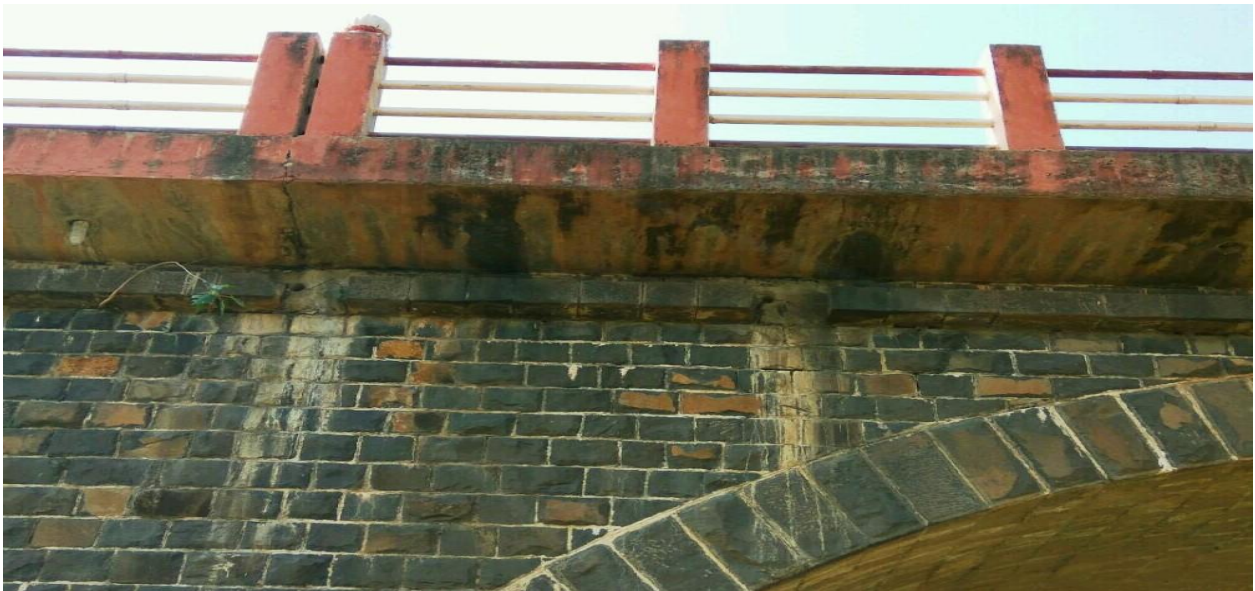
Fig 5: Photograph showing deteriorations above pier and outlet holes for drainage from deck.
