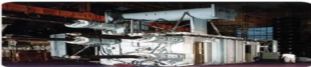
Fig 12 Transformer used for HVDC
