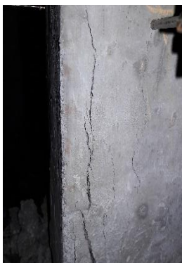
Fig5: NRC1 column Failure
