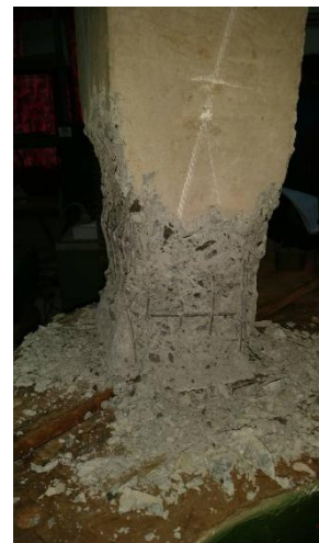
Fig10: CRC1c Column Failure
