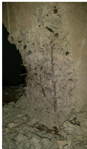
Fig9: CRC1b Column Failure
