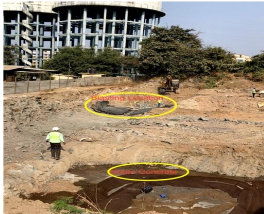
Fig 2: Freshly Poured Concrete near Blasting Sites at Mumbai Mumbra- Airoli Tunnel road work.
