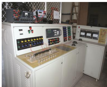
Fig 1: Power Supply Panel Board
