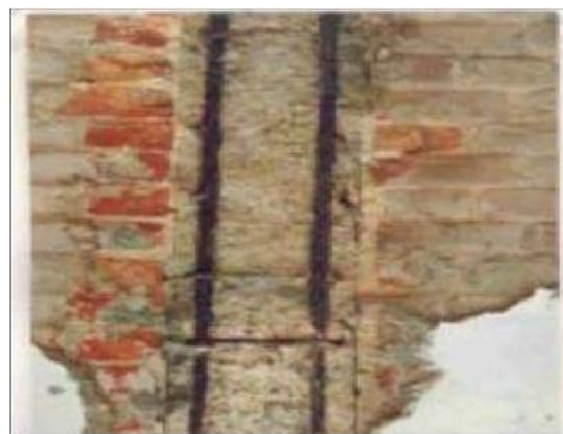
Fig. 02 Spelled cover concrete & exposed cover Reinforcement (Ref. Google)
