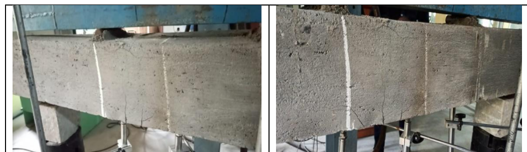
Fig 14 Failure and crack pattern of retrofitted RB2 beam
