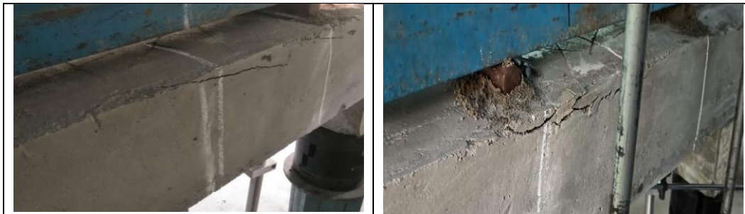
Fig 13 Failure and crack pattern of retrofitted RB1 beam
