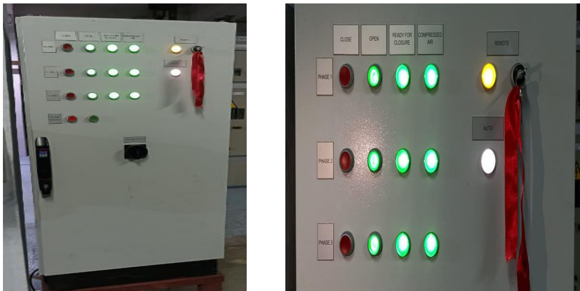
Fig.12 Local Control Cabinet (LCC)
