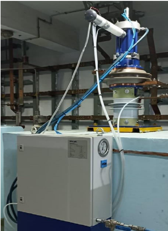
Fig.9 Make-Switch with Electro-pneumatic control cabinet (EPC).
