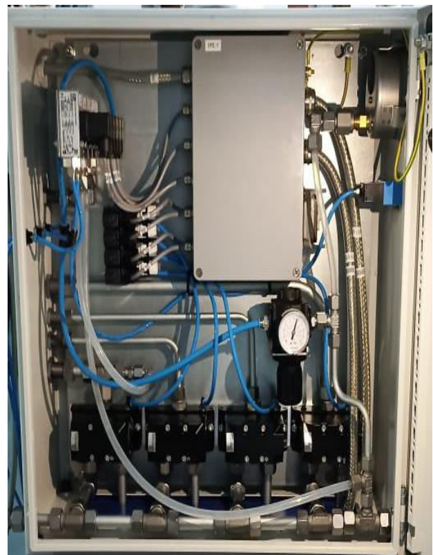
Fig.10 Inside view of Electro-pneumatic Control Cabinet (EPC).
