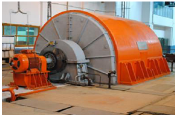
Fig. 3 1500MVA, 12.5kV, 69kA Short Circuit Generator with motor less excitation system (G2).
