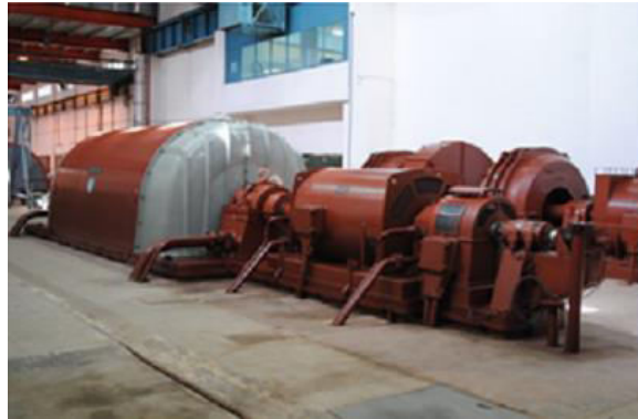
Fig.2 1500MVA, 69kA, 12.5kV Short Circuit Generator with DC generator excitation system (G1).
