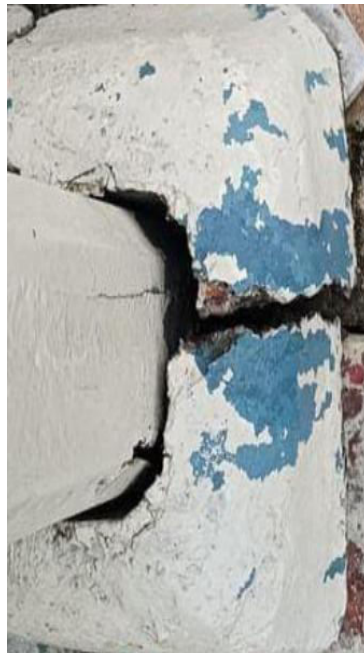
Figure 1:Crack more than 15mm
