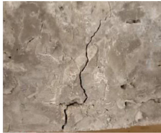
Fig. 11. Failure of beam
